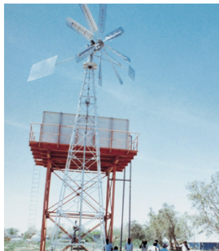
Figure 5. Locally-manufactured wind pump installed at kilo 8 site
