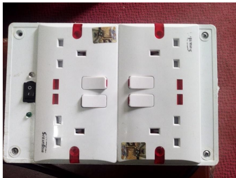
Figure 3.1. Distribution box and automatic change over relay
