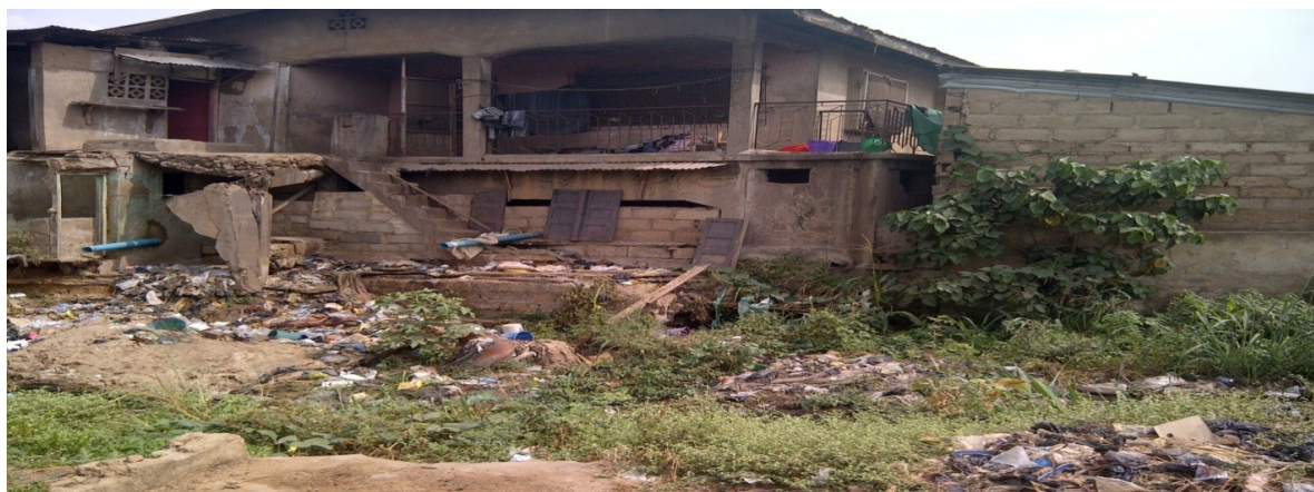
Figure 4.A building situated directly inside the Canal with Pipes from Toilet channeled Outside
