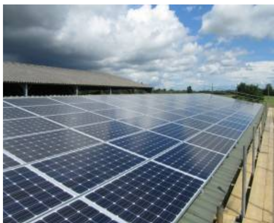
Figure 1. Typical Rooftop PV System: http://greentomatoenergy.com/case-studies-2/solar-case-studies/
